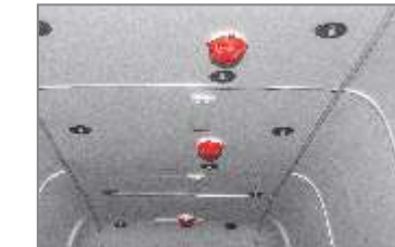
Water misting spray system covers all areas including windows, seats & sleeper berths
