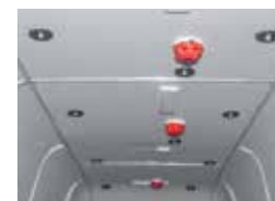
Water misting spray system
